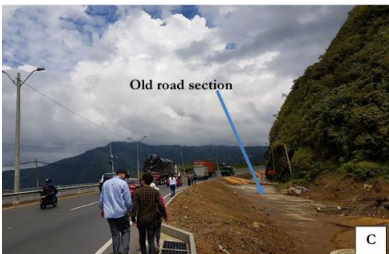
Figure 2.2: Representative landslides along the studied road section; A: Copacabana event 2016; B: Progressive downslope mass movement forcing authorities to divert the roadways and to construct tunnels; C: Large rockslide upslope causing traffic blockage
